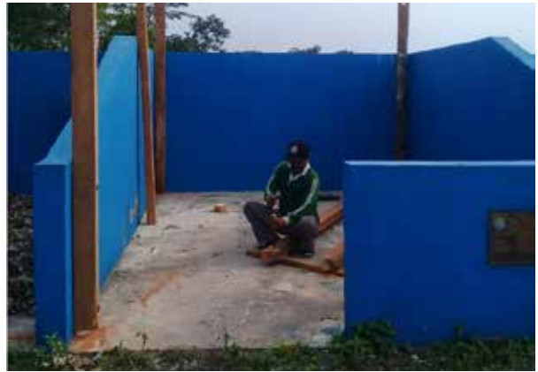
Supporting roof construction of temporary disposal sites (TPS 3R) in Depok village
