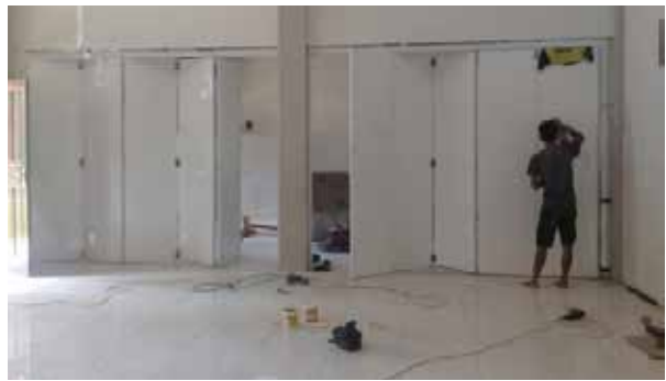
Support school infrastructure through producing room divider in Islamic boarding school of Jurang Jero in Bakalan village
